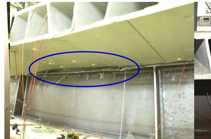
Failure of adhesive bond
