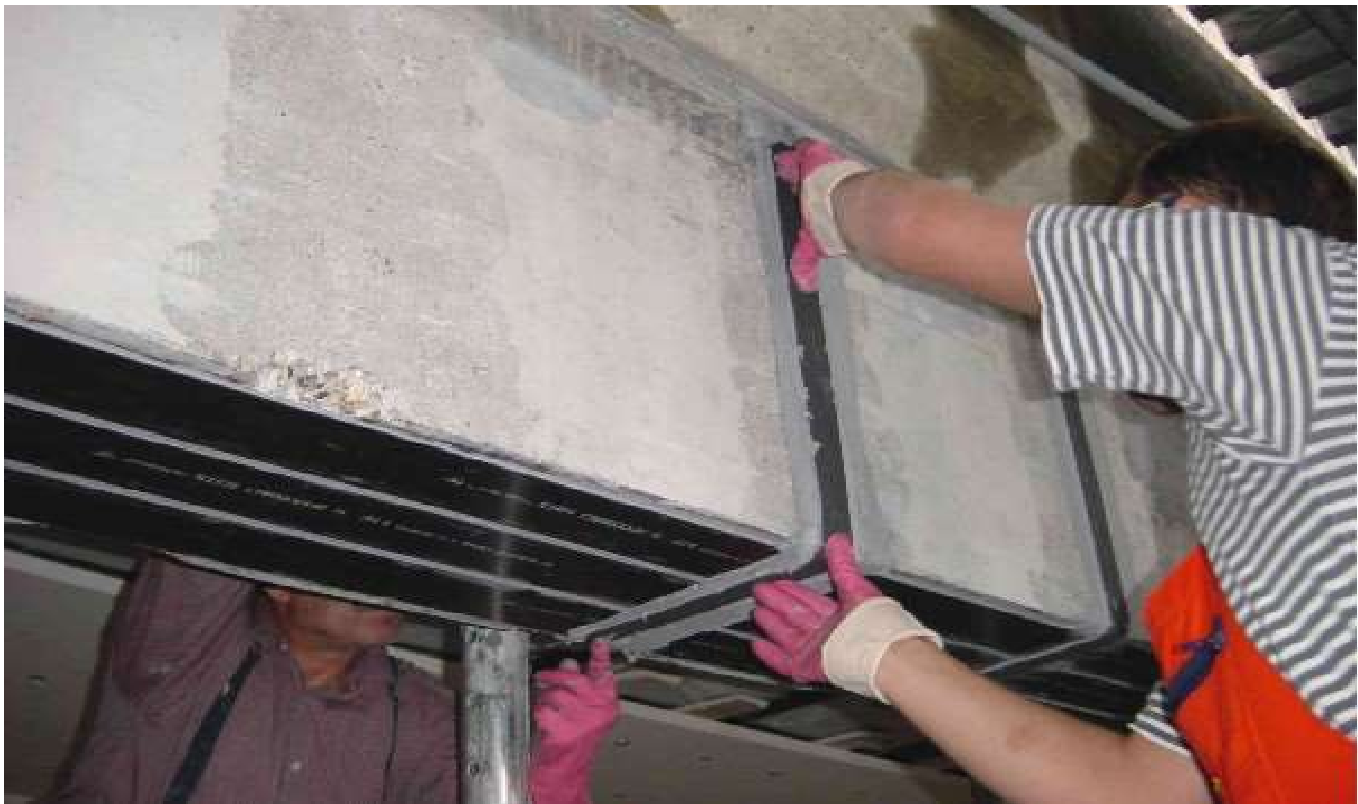
Installation of prefabricated CFRP L-shaped plates (shear strengthening) over existing CFRP strips (flexural strengthening)
