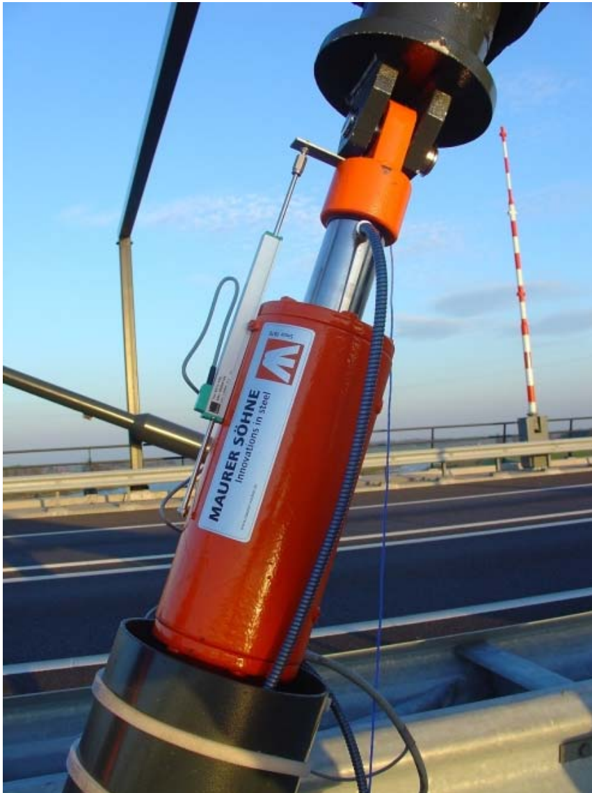
The magnetorheological fluid dampers are installed on the cable stayed bridge near Dubrovnik.
