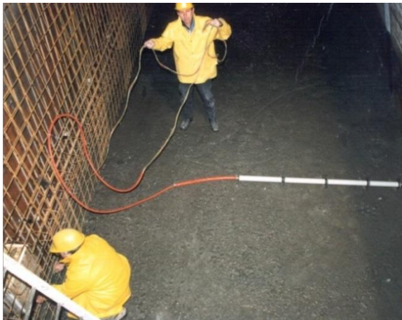
Power dam: Concrete-casting of an RSG sensor during the heightening of the dam in Luzzone, Switzerland.
