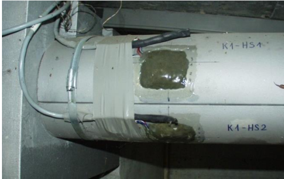
Bridge construction: RSG applied on the anchor head of a pre-stressed cable. Emmen, Switzerland.
