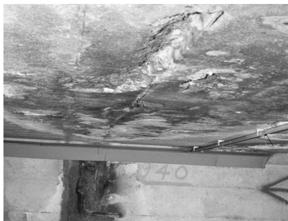
Figure 1: Deterioration of a concrete traffic plate at a joint promoted by de-icing agents due to failure of the waterproofing system in an alpine Swiss tunnel.
