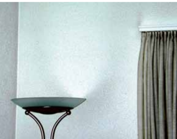
Typical damage in an apartment. The black staining is clearly visible.
